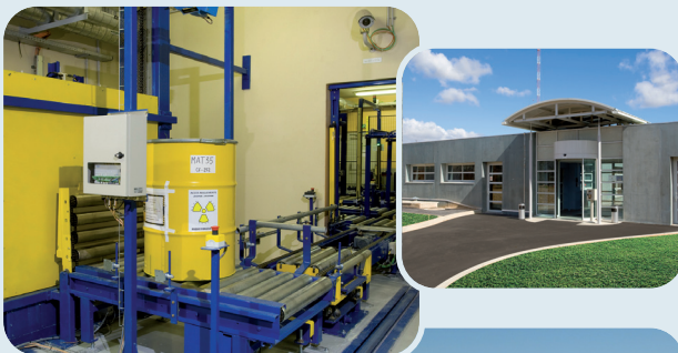
ROTONDE: the sorting and dispatching of low-level and very low-level waste packages
